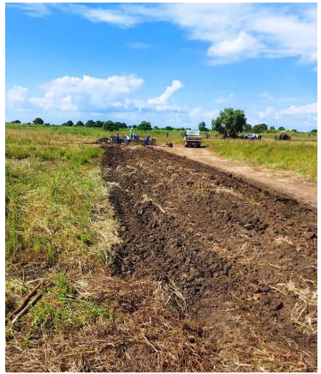
Foto 18: Field access roads need proper levelling and grading accordingly
