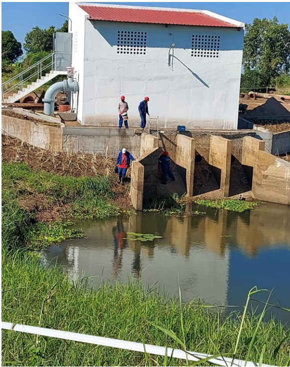
Foto 5: Pump house at the river
